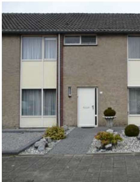
44. Double layered brick masonry with timber framed window element, 10 cm, poor insulation standard, NL-Roosendaal
