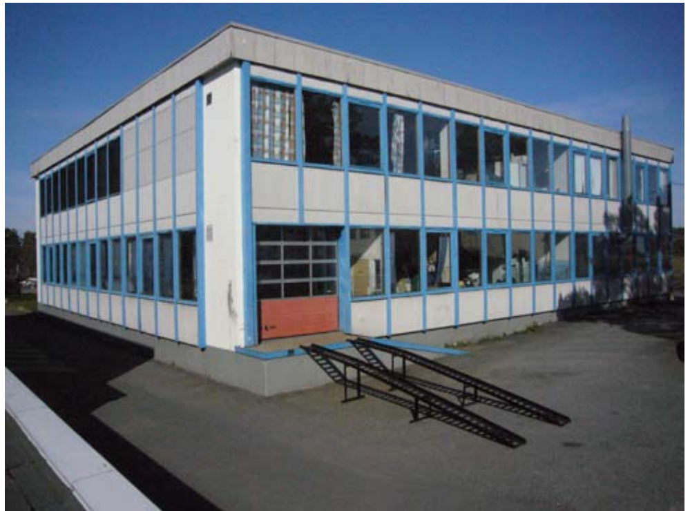
50. Timber frame wall with poor insulation, large window areas, NOR- Rsiør, College
