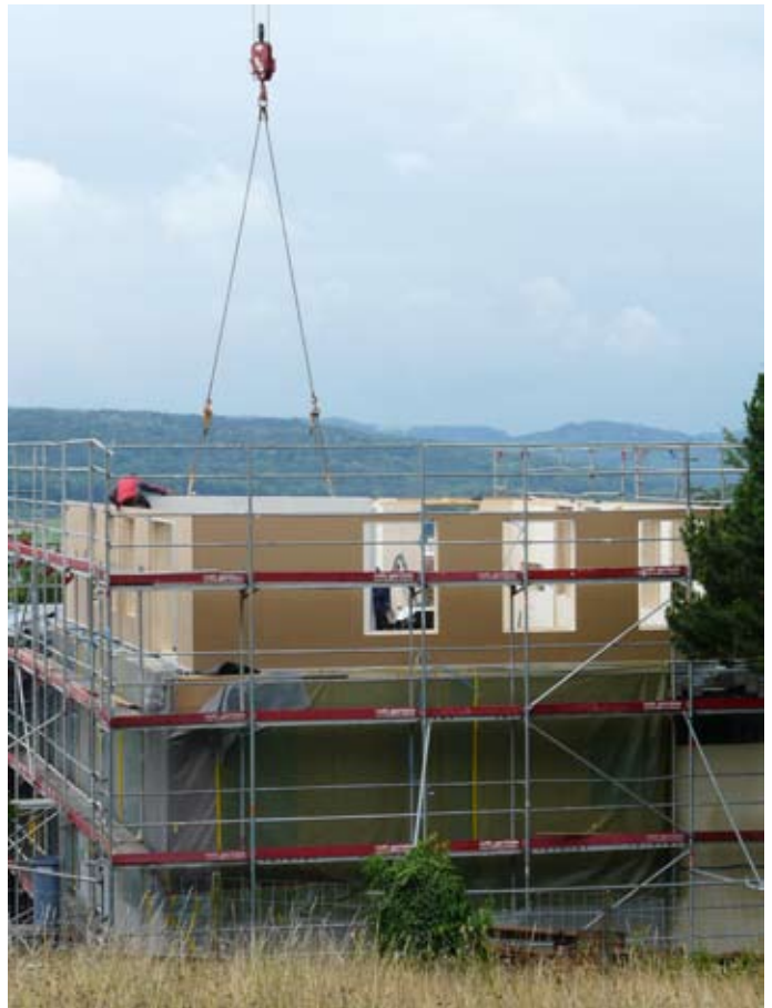
169. View from north: The extra top floor enjoys a spectacular view over Zurich and the mountains. The expected rent income „finances“ the modernisation of the whole project
