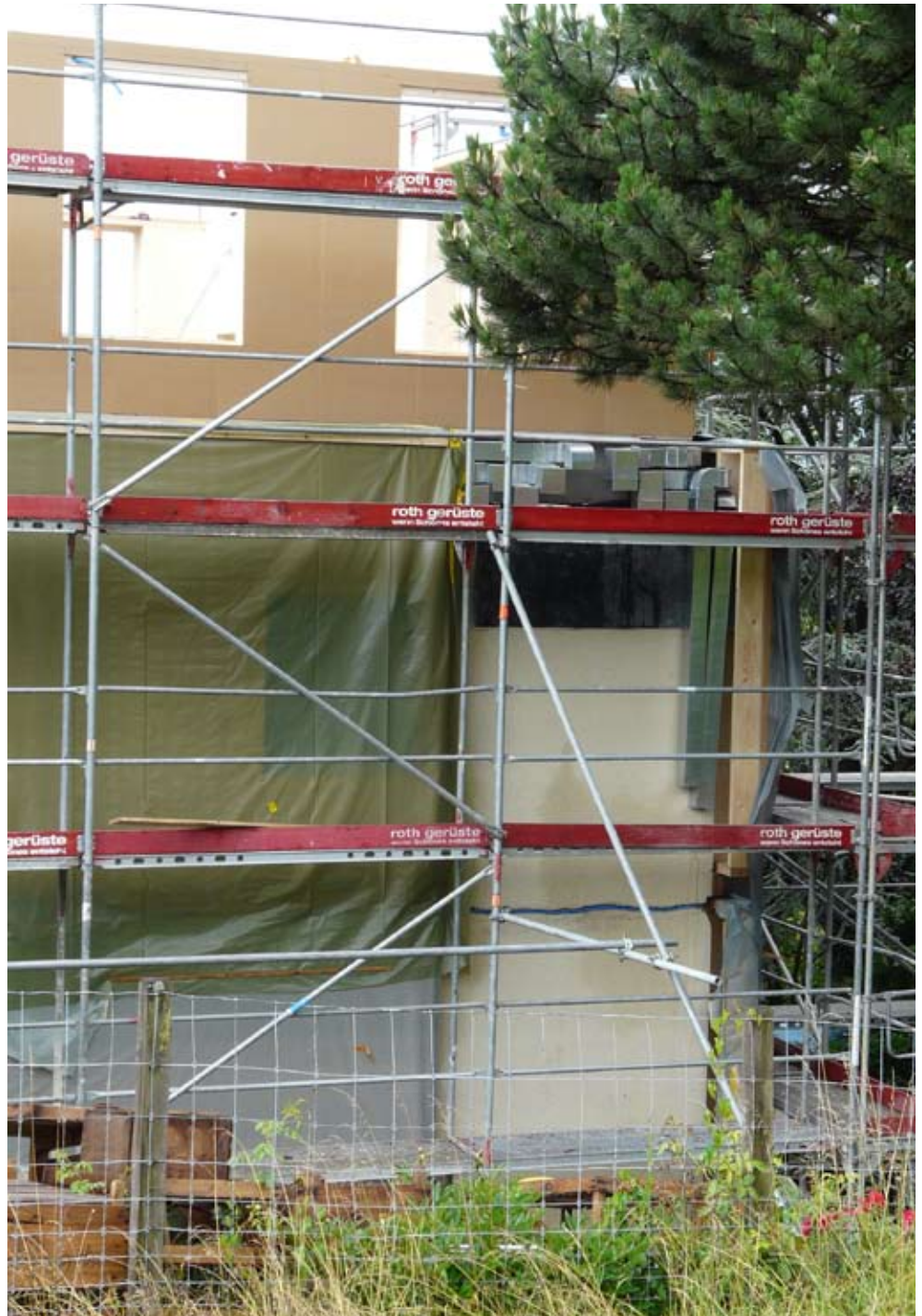
175. Weather protect elements (left) and HVAC routing vertical (right) and horizontal (top right).
