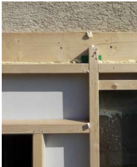
112. Joints sealed with PU foam.
