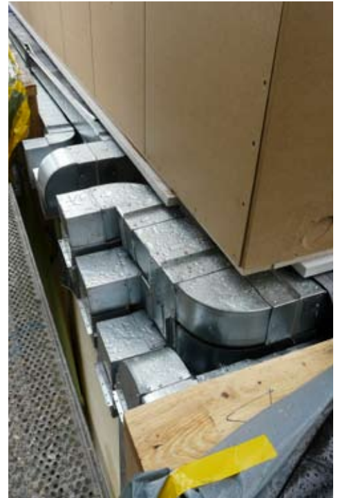
177. View of the bundle of pipes leading down into the central HVAC space
