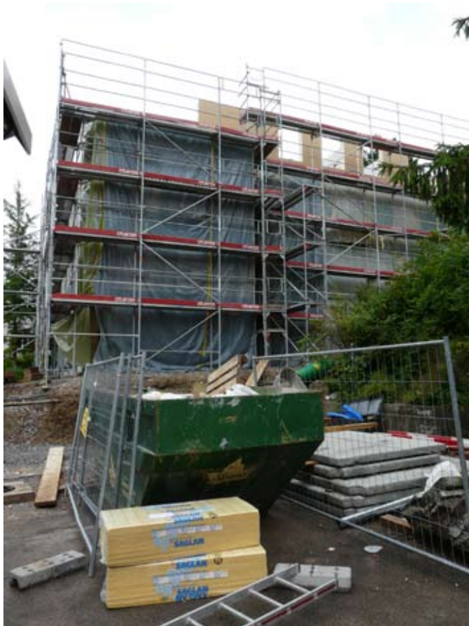
168. View from east (street side): the green plastic sheeting protects the new elements
