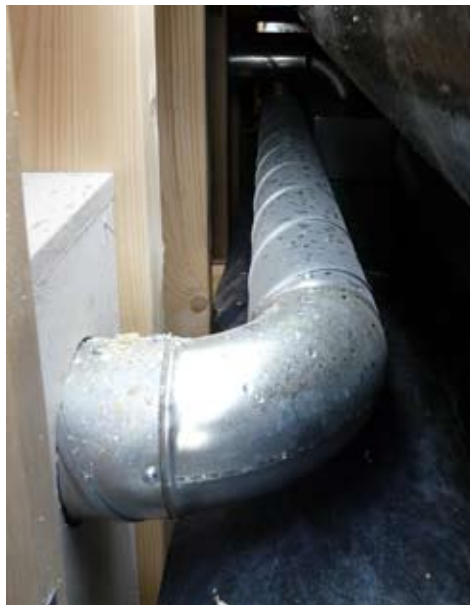
178. View into the setback. Transformation from horizontal to vertical pipe leading. This pipe is connected a lower floor.
