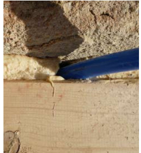
108. Insulation perforated by hose
