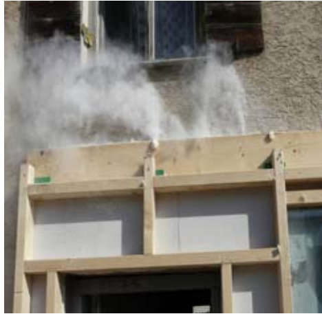
114. Dust emission through boreholes.
