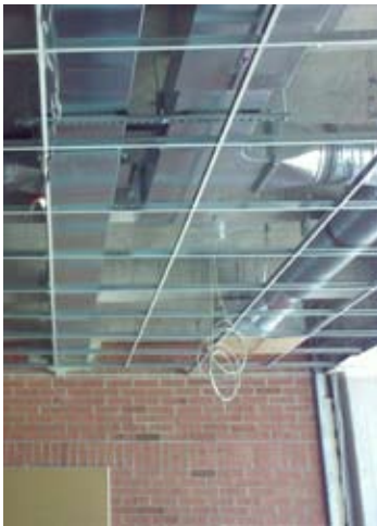
198. New ventilation system in the suspended ceiling
