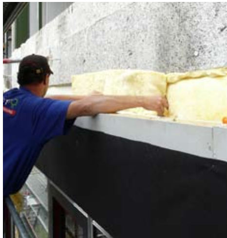
101. Fixation of adaption layer on the existing wall. Depicted here is a Heraklith surface, Real-schule Buchloe
