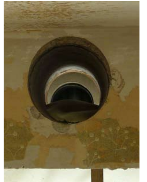
179. Pipe lead through above a window
