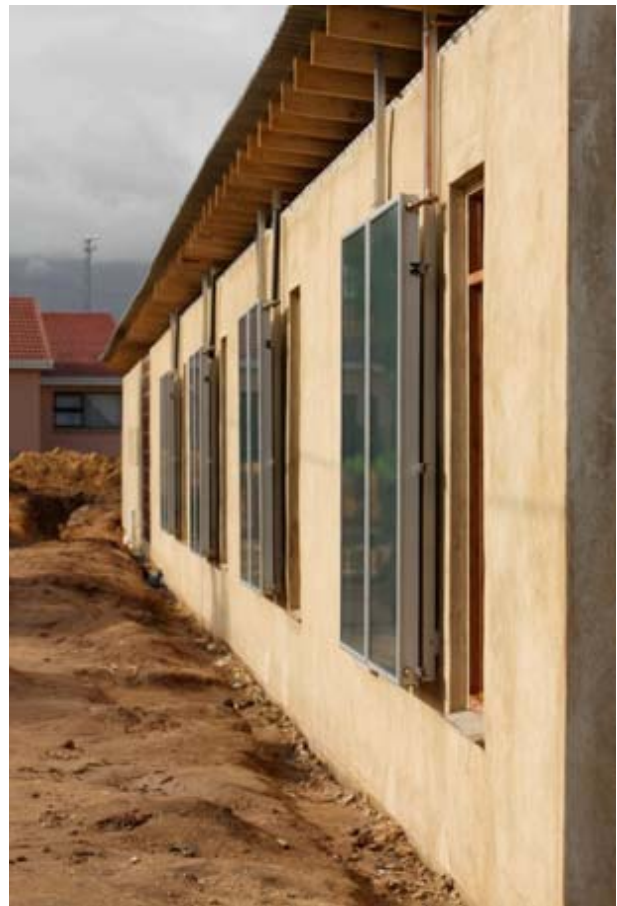
Figure 14: solar panels on North facade
