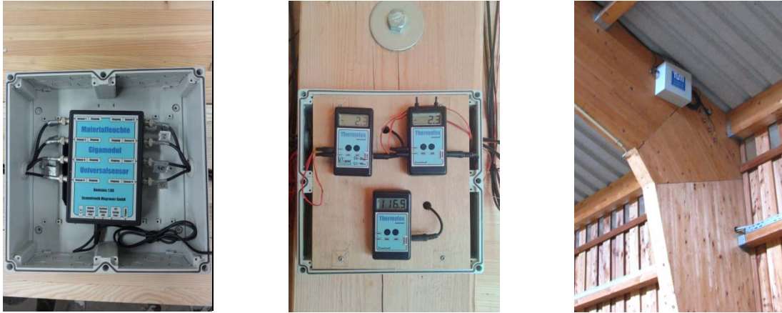
Figs. 18-20: Examples of measurement system installed on site, from [17], [18]
