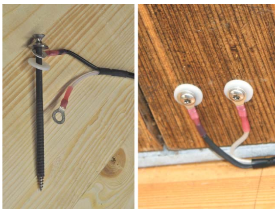
Fig. 15: Example for screw-type electrodes before installation and installed on-site, from [19]
