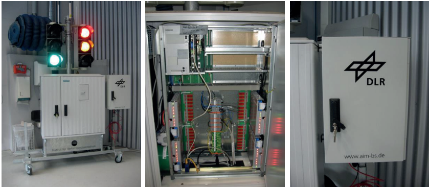
Figure 2: Field operational test installation (left) with the signal controller Siemens C940V (middle) and the road side unit (right).
