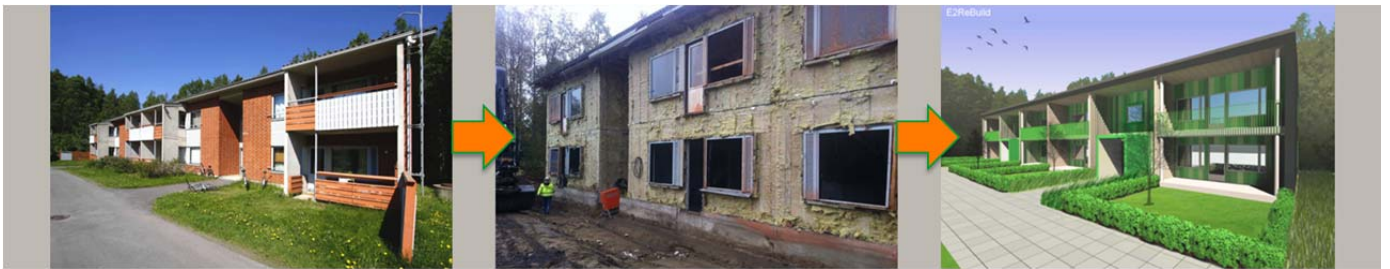
Figure 2-25 Process of change from original building, refurbishment site process, to end result at E2ReBuild demonstration project PSOAS Oulu (photos M3 Architects, le Roux)
