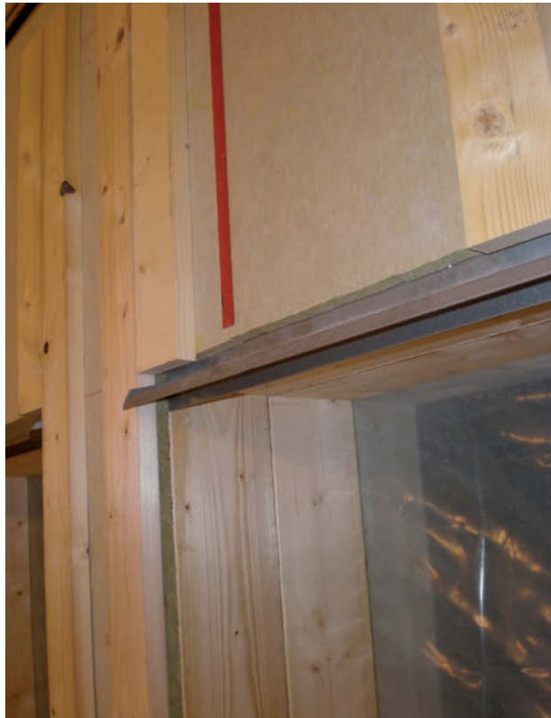
F7.5 Mould-resistant insulation board protecting the studs and a two-step tightened façade with a well-ventilated drainage layer behind the cladding.
