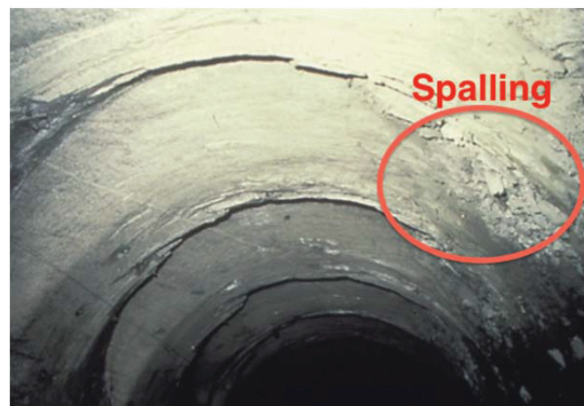
Fig. 9: Overbreak due to what was described as spalling and crushing at Kobbelv. Modified from MYRVANG et al. (1998).
