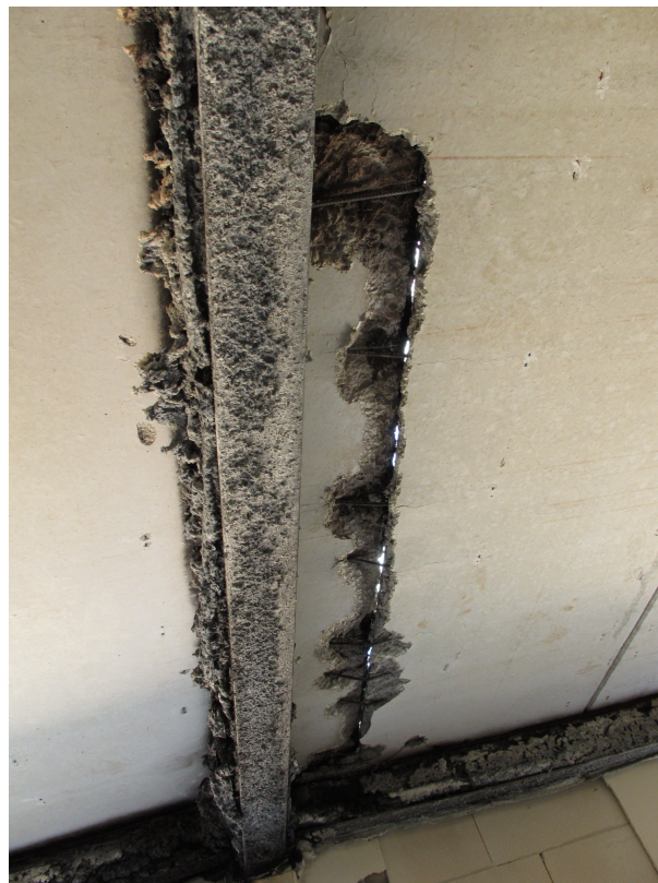
Fig. 3.10: View from below at gaping crack at first Munich test according to [42]
