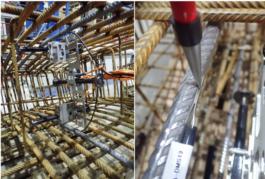
FIGURE 6 Instrumentation details U5; left: vibrating wire sensor, right: welded strain gauge.
