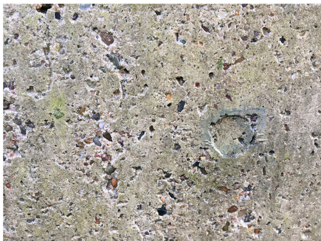
Figure 1. Surface deterioration of a concrete wall with a high saturation freezing and thawing exposure at a floodgate in Germany.
