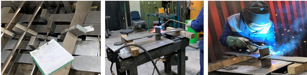
Figure 4-1: Staped test specimens before the welding process (left) preheating process to reduce welding residual stresses (middle) and welding process (right)
