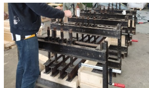
Figure 18. Lamination process of the timber structure of an M-series prototype using a spindle press and IPE100 beams.
