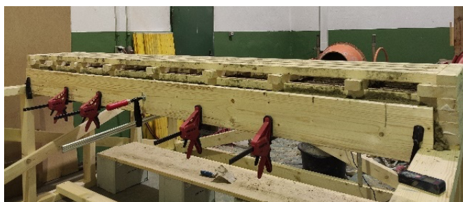
Figure 17. Casting Process of an M prototype. Bottom and side formwork are directly connected to the timber structure using screws and clamps, and the arrangement is not supported in the centre, to allow for bending already during the casting process.
