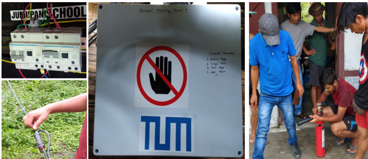
Figure 13.16: Safety installation. From the left, RCBOs, IP68-rated wire connectors, warning stickers and fire extinguisher.[93].
