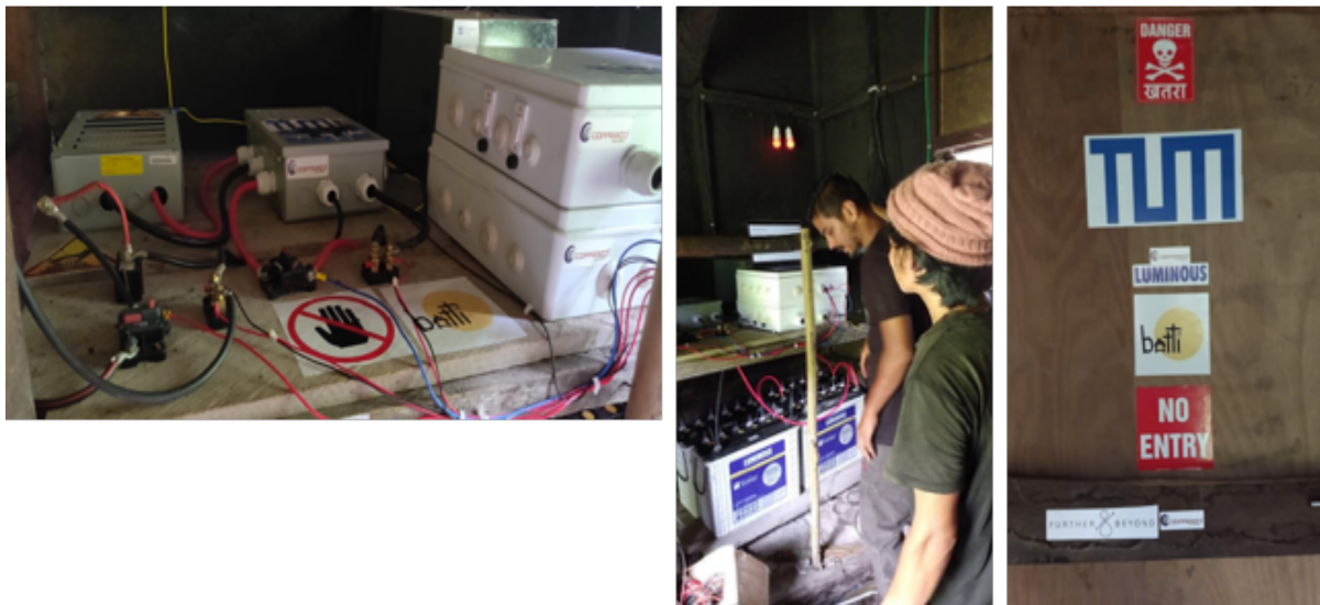
Figure 13.7: Interfacing components and battery bank installed into the control room.[93].
