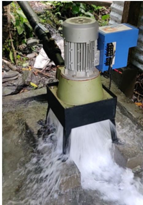
Figure 13.5: The turgo turbine after installation.[93].
