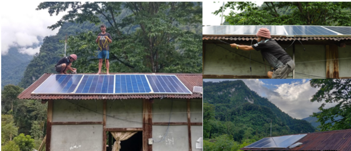
Figure 13.2: PV installation on the control room rooftop.[93].
