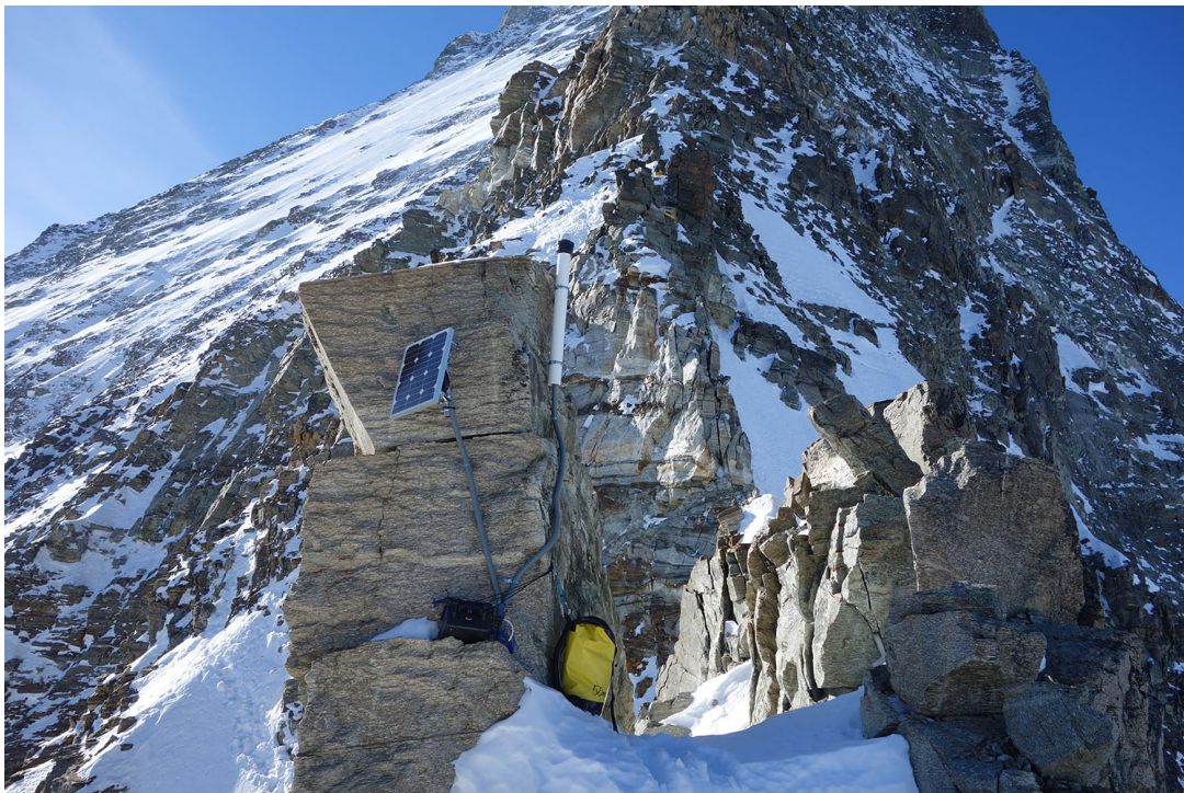
Figure C10. Wireless L1-GPS installed at position MH34 monitoring the gradual tilting of a little tower feature that is separated from the main ridge.
