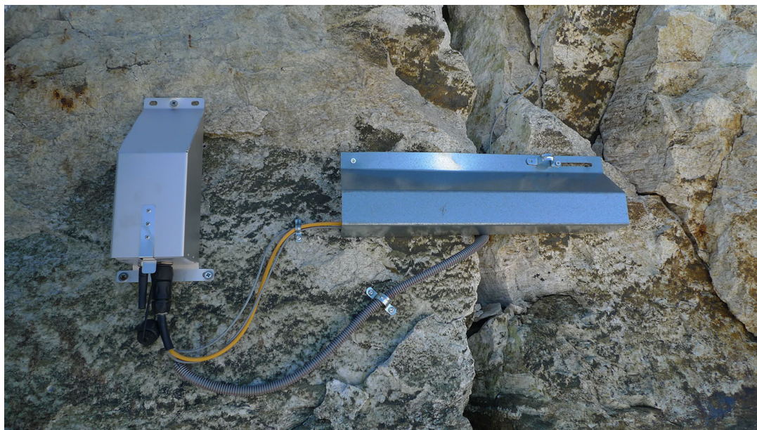
Figure C5. Close-up of crackmeter and thermistor chain installation at position MH03. The wireless sensor node is housed in the steel protective shoe on the left while the crackmeter is located under the steel protective shield in the middle.
