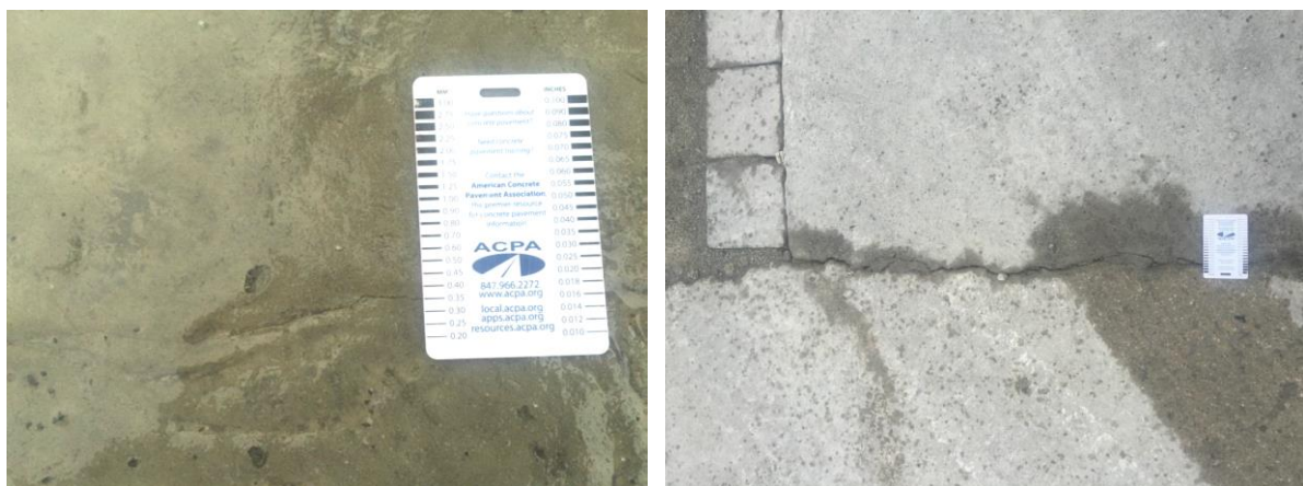
Figure 8.15 Cracks on first trial cast in situ of ECC-Cor
