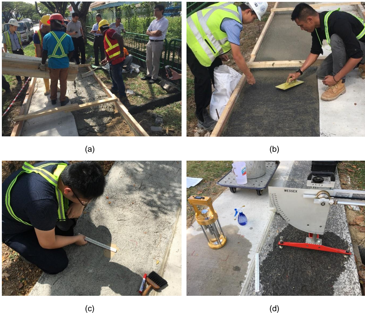
Figure 8.5 Spreading aggregates onto ECC for footpath application (a) casting normal ECC, (b) spreading aggregates onto ECC surface, (c) SPM test, and (d) BPT test
