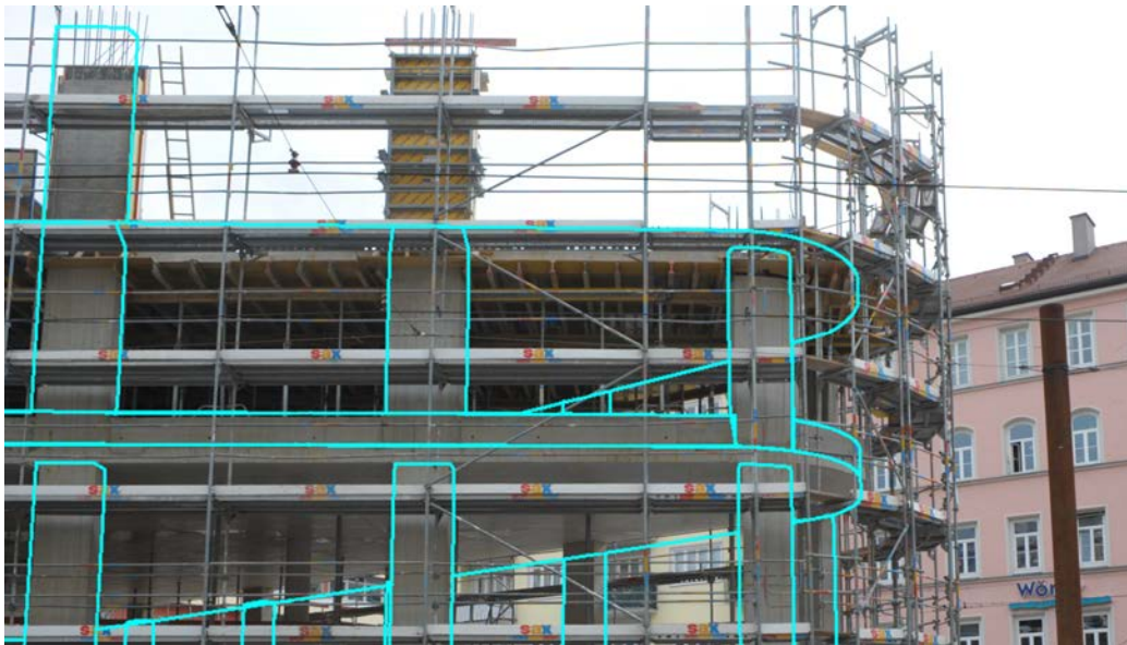
Figure 11: Sample sub-set of auto-labeled columns and walls in another picture from a construction site.
