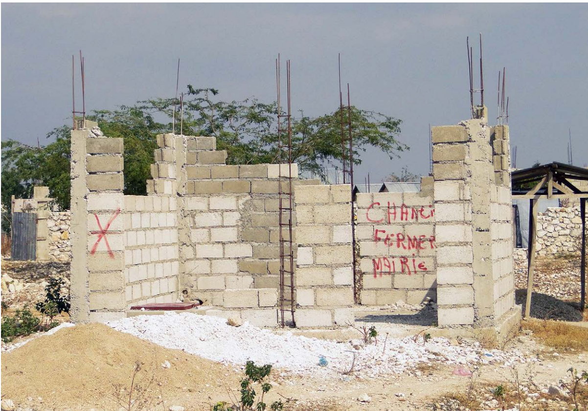
Fig. 46: Construction site closed by the local authority Thomazeau
