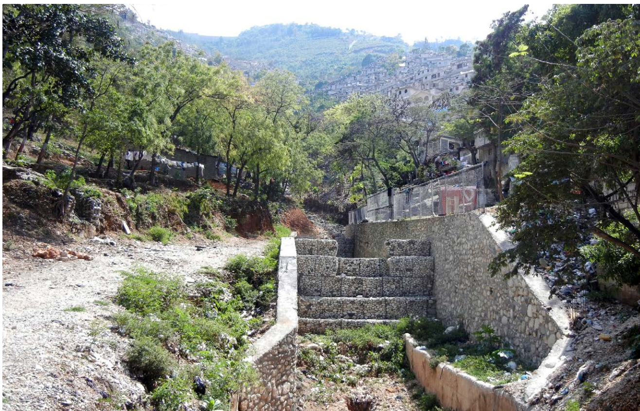
Fig. 32: Ravine with basins for debris load retention in a Morne l'Hôpital neighborhood, Port-au-Prince
