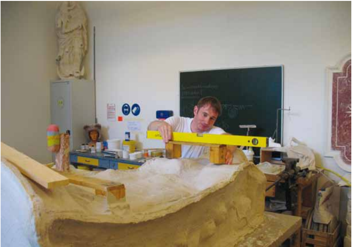
German-Chinese team repairing the wall murals in Beiwusheng huiguan The village of Wafangdian with the Beiwusheng huiguan near Ziyang The molding and manufacture of the plaster model
