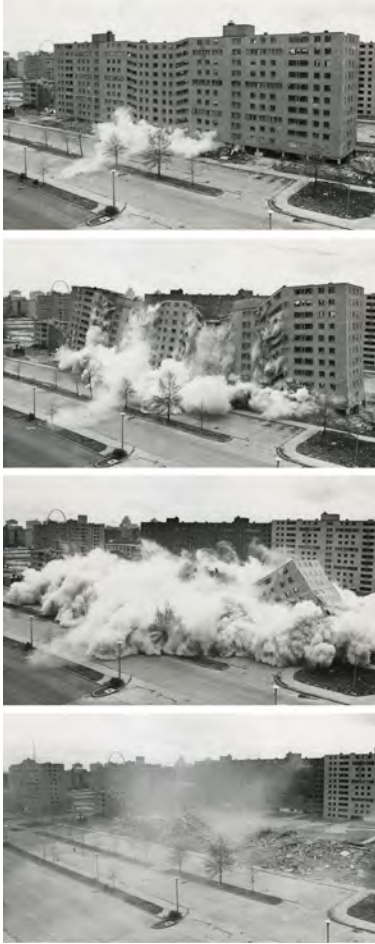
Figure 3.1: Pruitt-Igoe Collapse Series, April 1972. The second, widely televised demolition of a Pruitt-Igoe building that followed the March 16 demolition. Pruitt-Igoe was a large urban housing project located in American city of St. Louis. It was also the first large independent work designed by Architect Minoru Yamasaki. Soon after its completion in 1956, living conditions in Pruitt-Igoe began to decline. By the late 1960s, the complex had become internationally infamous for its poverty, crime, and segregation. Its 33 buildings were torn down in the mid-1970s. The event has been viewed by theorist Charles Jencks as an icon of modernism's death. See "Pruitt-Igoe," last modified May 04, 2013, http://en.wikipedia.org/wiki/File:Pruitt-igoe_collapse_series.jpg .
