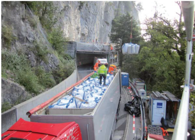
Abb. 12: Anlieferung der Schaumglasschotter Module per LKW. Fig. 12: Delivery of the damping moduls by truck.
