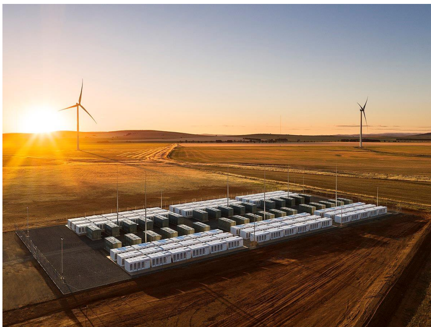
Figure 4. Hornsdale Power Reserve in South Australia. The grid-connected battery energy storage system provides a capacity of 193.5 MWh at 150 MW. Picture reproduced from ref. 52.
