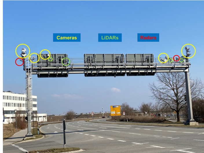
Figure 5.28: One of the measurement points of the Providentia++ project on the A9 highway ( https://innovation-mobility.com/en/project-providentia/a9-dataset/ ). The A9 dataset [Cre+22] is obtained from roadside sensors, including multiple LiDARs, cameras, and radars.
