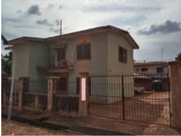
Fig. 1 A residential housing in the Abakpa housing property in Enugu with decaying roof, windows and weakening fence walls
