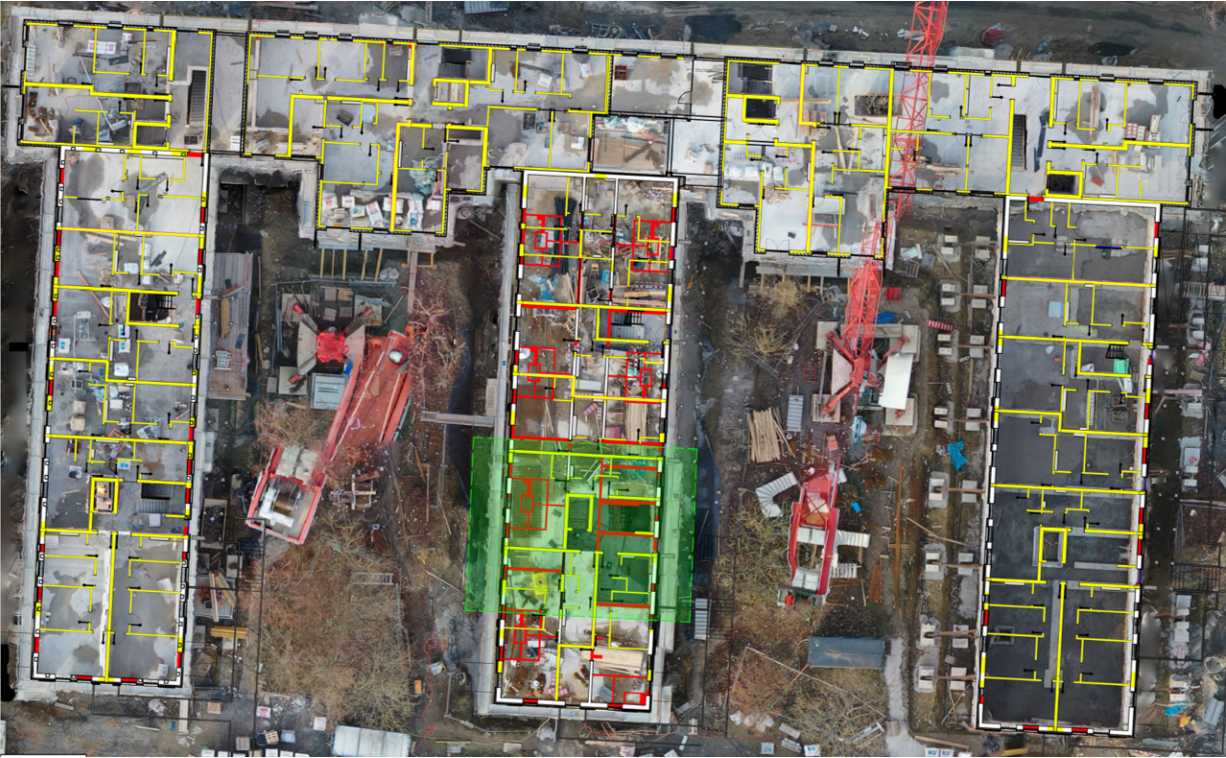
Figure 6.3: Construction site: UAV based orthomosaic (top view) augmented with planning data as overview of the construction site of scenario 2 (indoor conversion). The project mainly involves the demolition of existing walls (red) and the building of new walls (yellow) for new room layouts. The green rectangle indicates the study area for which as-built measurements were conducted.
