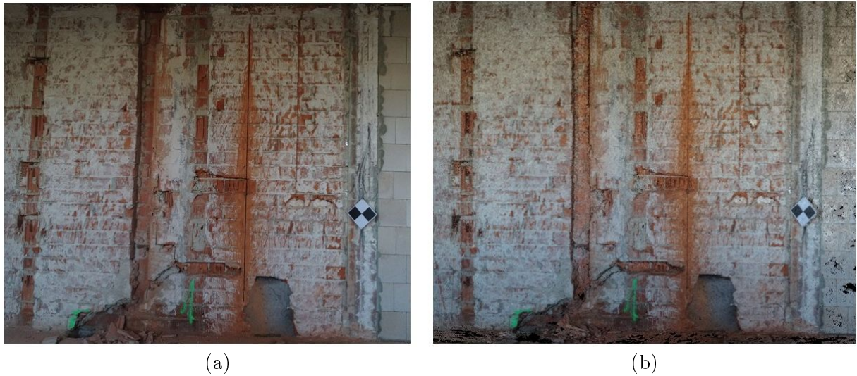
Figure 6.7: Exemplary sample of a TLS cloud (a) and a corresponding photogrammetric dense cloud (b) of a brick wall from scenario 2
