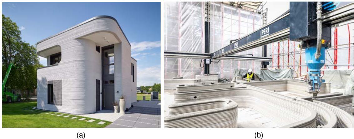
Figure 1.1: 3D printed residential building in Beckum finished (a) (PERI®, 2021) and under construction (b) (PERI®, 2020)
