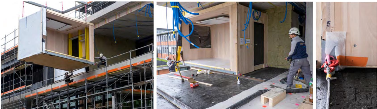
Figure 299 – Example of assembly procedures of wooden prefabricated boxes from NEST (EMPA, CH) – Source: [211]
