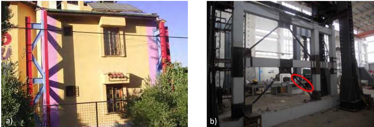
Figure 18 – a) Buttress type external steel wall; b) RC frame strengthened with steel braces – Source: [27, 34]
