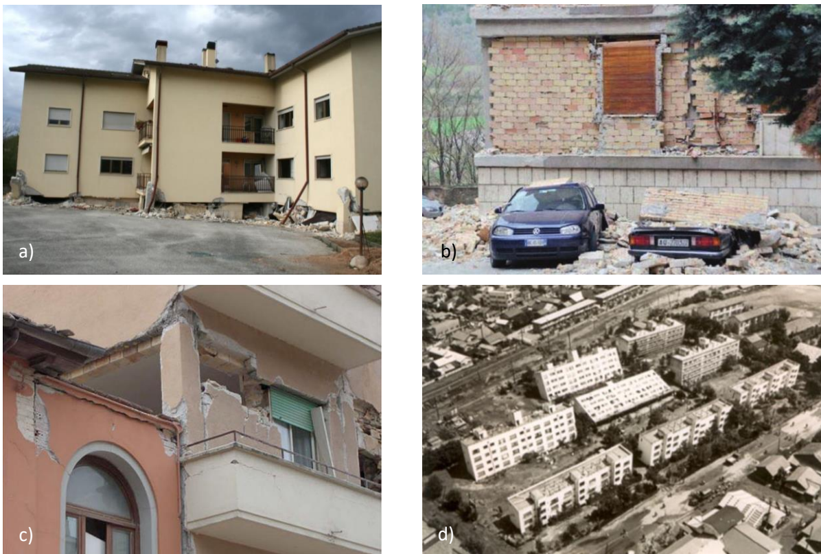
Figure 5 – a) Example of soft storey mechanism in L’Aquila (Italy), 2009; b) ejection of the external panel and bending collapse of the interior one; c) pounding between new and old building in L’Aquila (Italy), 2009; d) Overturning residential building in Niigata City (Japan) due to liquefaction of sandy soil in 1964 – Source: [9, 19-21]
