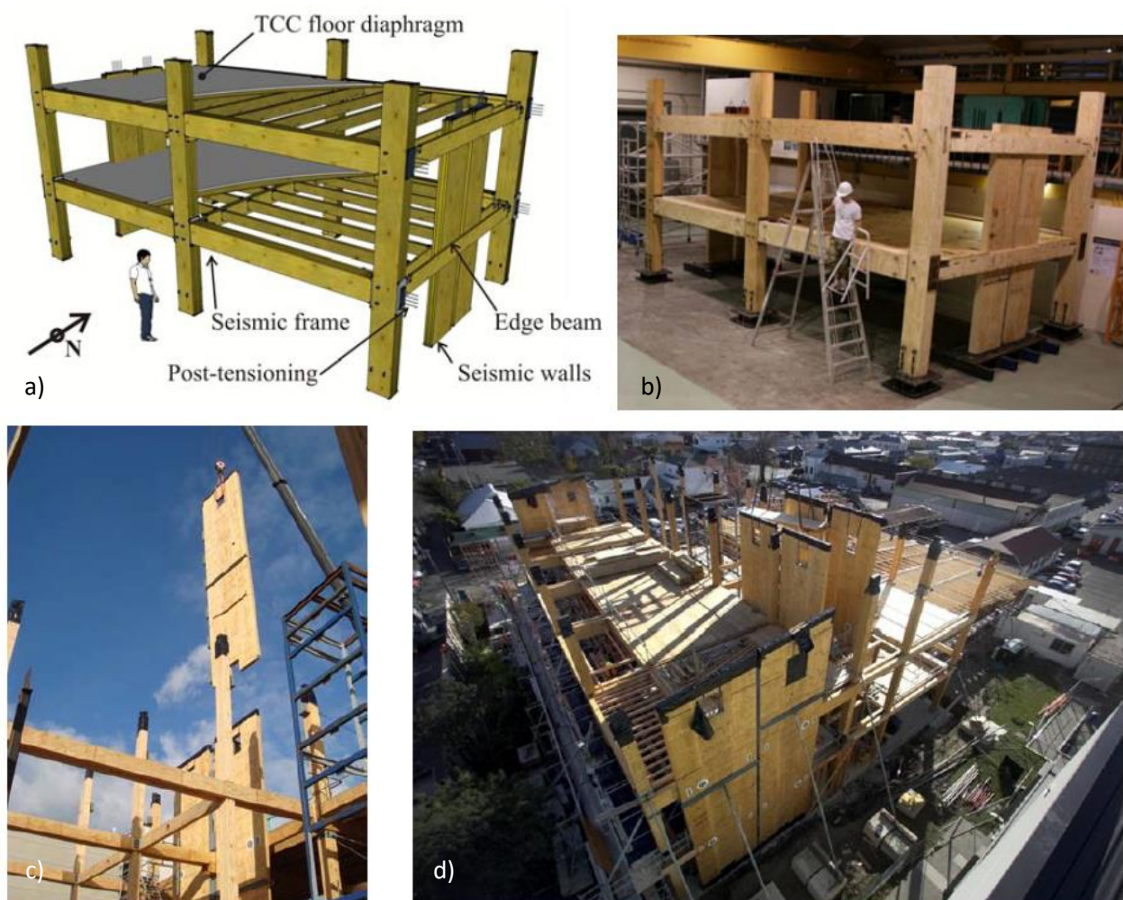
Figure 213 – a) Isotropic view of the test building presented by M. P. Newcombe; b) photo of the test building presented by M. P. Newcombe; c) and d) photos during the construction of the NMIT Arts & Media Building – Source: [190, 194]
