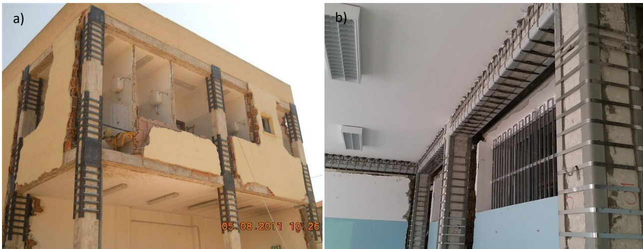
Figure 8 – Steel jacking of existing reinforced concrete members. a) A traditional approach; b) the CAM system – Source: [29, 30]
