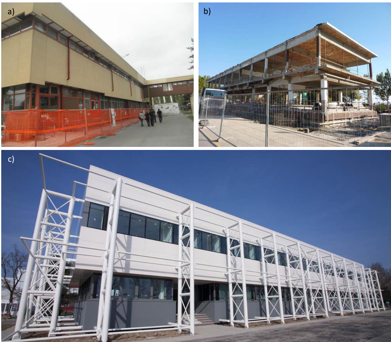
Figure 54 – a) Photo of the building before the intervention; b) photo of the RC bearing structure and realisation of the Mesnager hinges; c) photo of the building after the renovation – Source: [109]
