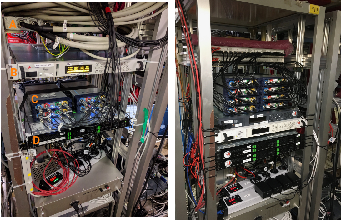
Figure A.1: Phase 2 (left) and 3 (right) DAQ hardware. The data acquisition system in the electronics hut. Reading the orange numbers on the left: The patch panel (A) connects to a Keysight N6700 power supply (B) and the dock box providing three different voltages. Four PicoScope 6404D oscilloscopes (C) digitize the analog SiPM signals and transmit them to the custom made C++DAQ software on the working machine (D).
