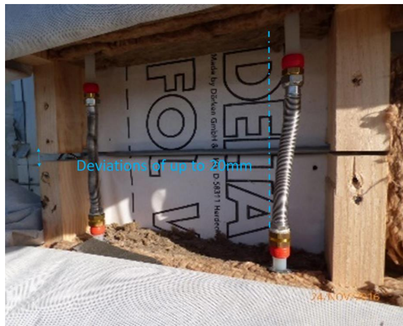
Figure 23: Deviations appeared during the installation of the modules.
