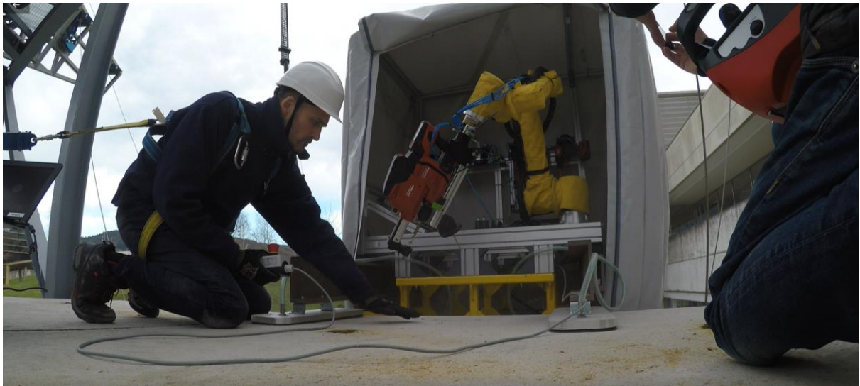
Figure 78: The MEE in operation [119]. Pictures by Julen Astudillo (Tecnalia).
