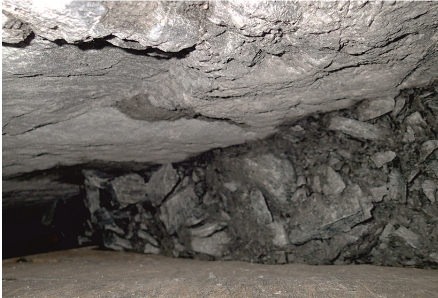
Fig. 100: Accumulation of rock debris in the area between the cutter head and the tunnel face.
