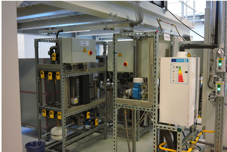
Figure C.7: Overview about heat modules of SFH-2: Left background is the air heat pump, right foreground is the gas boiler, center left is the grid transfer station module.
