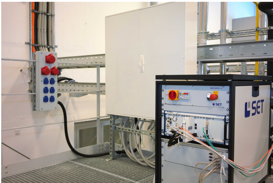
Figure C.5: Overview about electricity and control system of SFH-3: Left are the sockets, center is the house's electricity distribution cabinet, right is the RT control system.
