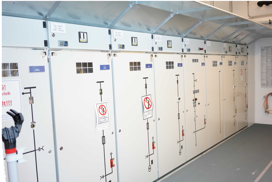
Figure C.1: View into the MV room
