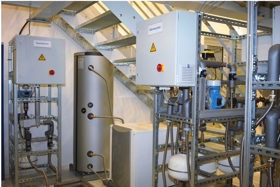
Figure C.9: Overview about the brine heat pump: Left center is the brine tank, center is the heat pump itself, right is the pipe circuitry.
