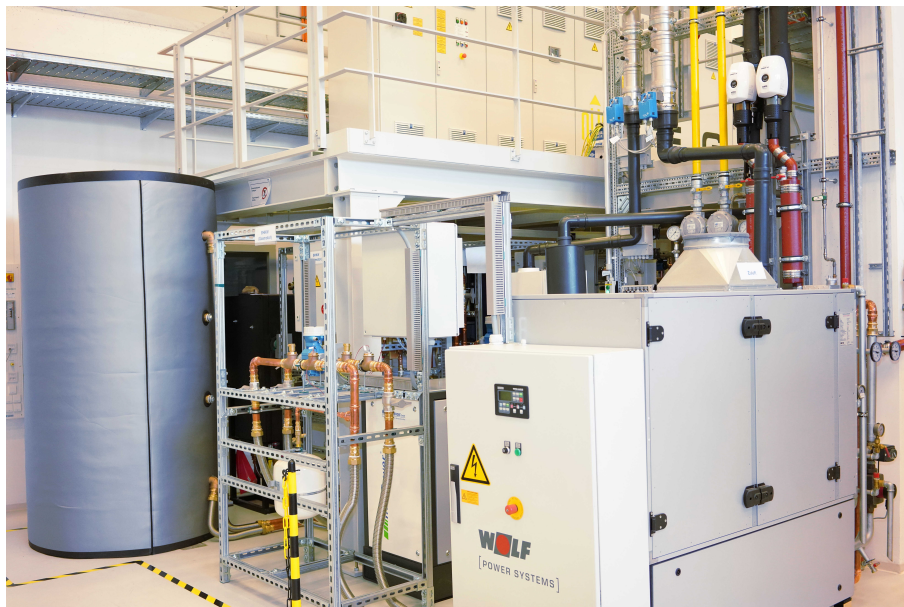
Figure C.8: Overview about heat modules of MFH: Left is the heat tank, right is the largest CHP, right top is the connection for exhaust, natural gas and cooling water (pipes without insulation).
