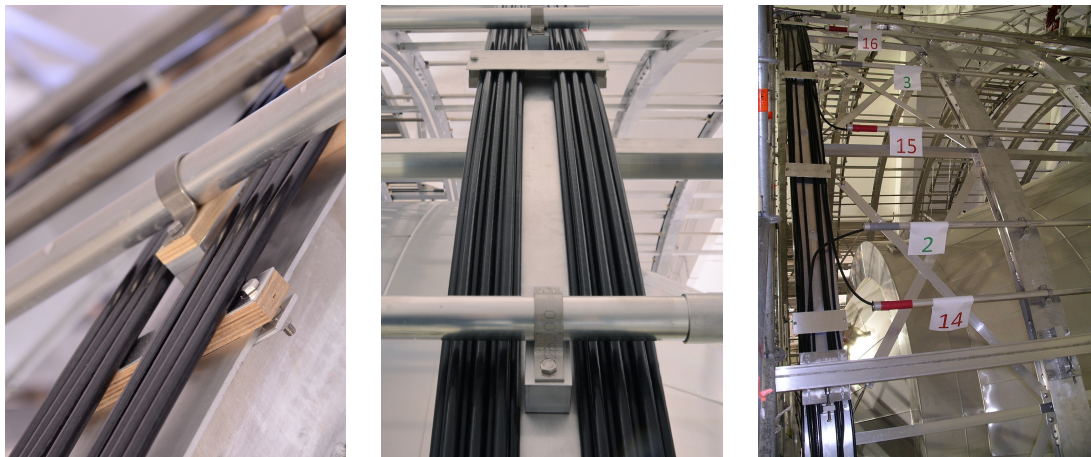
Figure 6. LFCS and EMCS cabling details. Left: 8-turn LFCS coil with wooden spacer and EMCS pipes running across. Middle: a 14-turn coil guiding 8 lower cables and 6 cables on top. Right: EMCS loops are completed on the end rings. The vertical correction (horizontal loops) is marked by red numbers, the horizontal correction (vertical loops) by green numbers.
