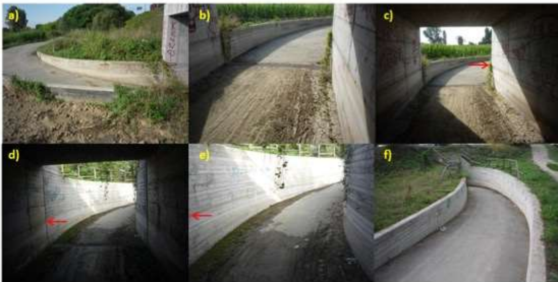
Figure 6. Poor design, worse construction: the Binasco underpass connecting two portions of the bicycle rout flanking the Naviglio Pavese
