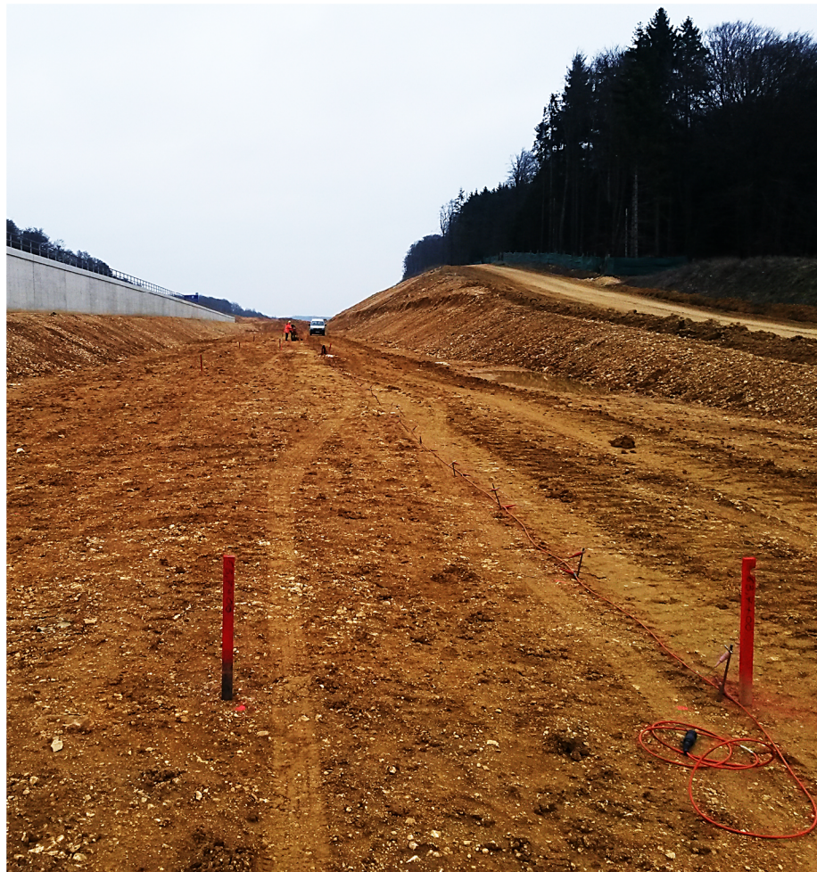
Fig. 24: Photograph of the 2D ERT survey layout, with one 320 m long profile (2.0 m inter-electrode spacing, 120 m maximum field layout) along the southwestern line track (direction Stuttgart to Ulm).
