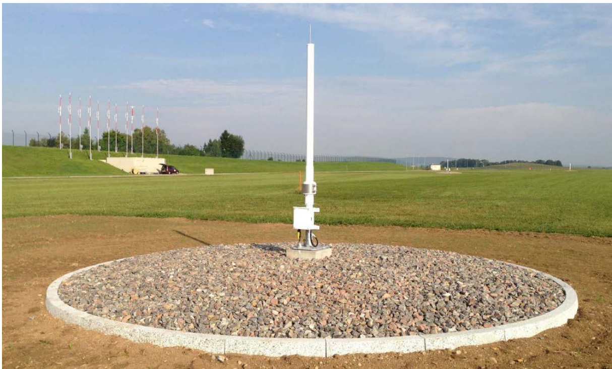
Figure 2 GBAS reference antenna at Zürich Airport (LSZH) [28]
