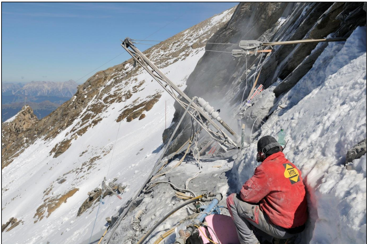
Figure 34: Air flush rotary drilling at the Kitzsteinhorn west face in September 2010 (borehole depth 30 m) (Photograph by Ingo Hartmeyer).
