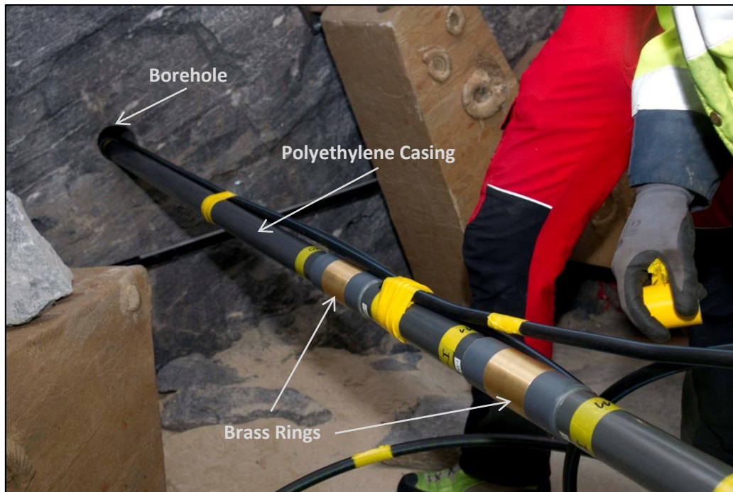
Figure 35: Borehole instrumentation inside the 'Hanna-Stollen' with a purpose-built temperature measurement system developed by GEODATA ZT GmbH (December 2011). The black tube serves to fill up the annulus with concrete after the insertion (Photograph by Robert Delleske).
