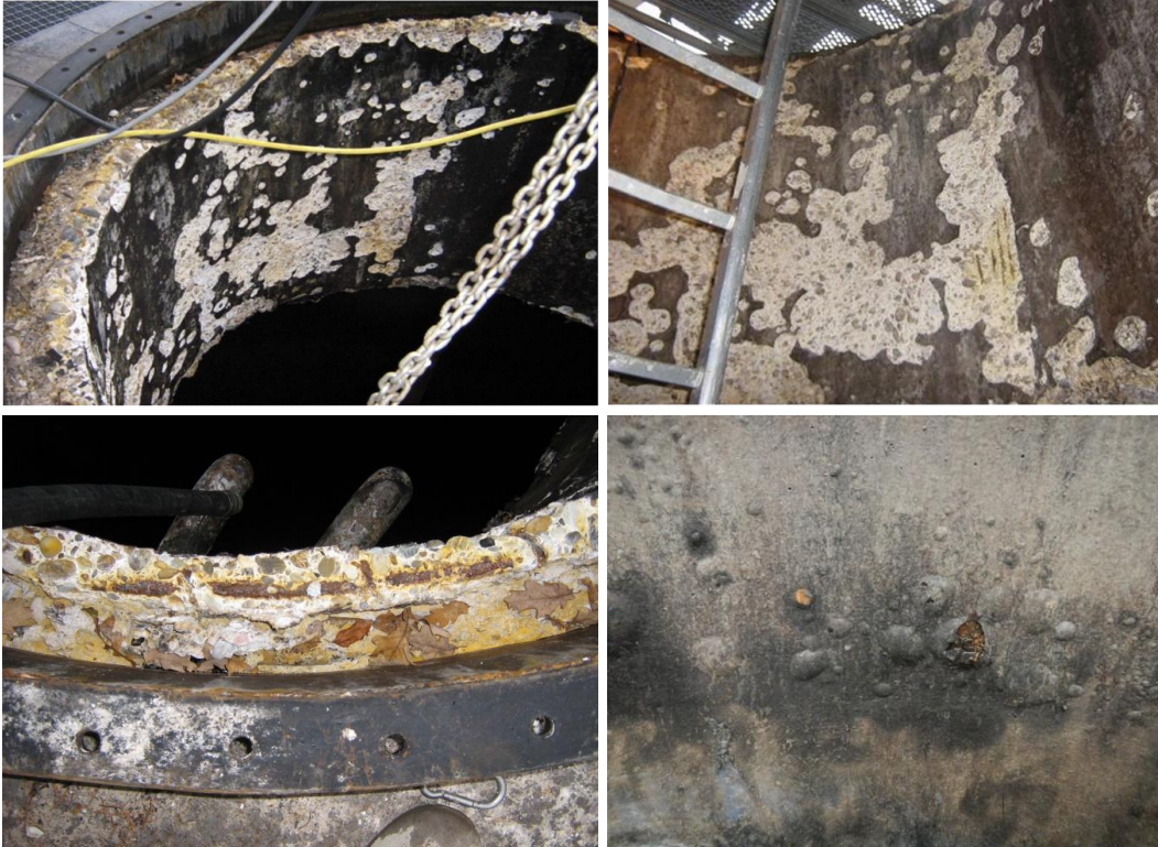
Figure 1.4 Severe concrete corrosion observed within the headspace of two different digesters in Germany. © Weber-Ingenieure GmbH.
