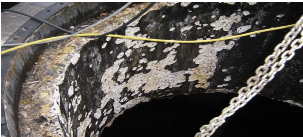
Figure 4.1 Concrete corrosion pattern observed in the headspace of digester E.
