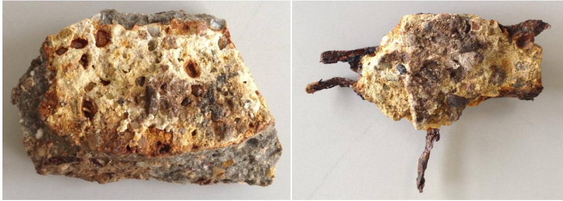
Figure 1.3 A heavily corroded piece of concrete originating from a sewer pipe in Germany. © Bettina Huber
