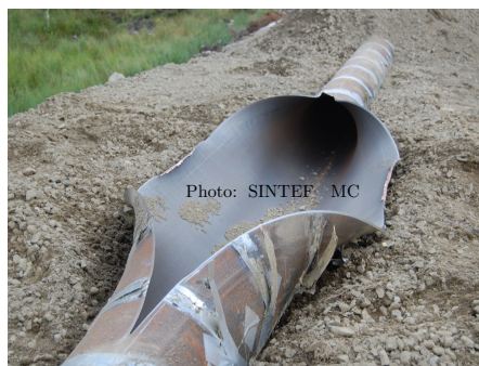
Fracture of liquid carrying pipeline
