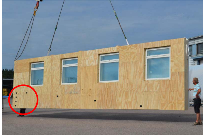
Figure 1-1 TES Element with integrated ventilation ductwork. The element is handled horizontally but will be turned to vertical orientation on-site. [Lylykangas]
