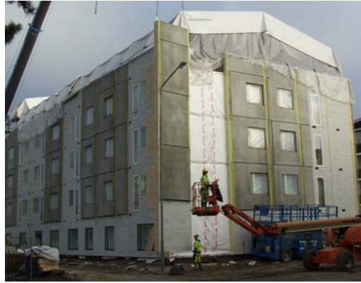
Figure 1-44 Construction site assembly of prefabricated elements with first render layer [Paroc Group Oy].
