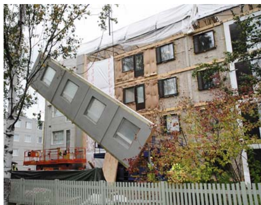
Figure 1-45 Turning of elements from truck into the vertical position for assembly [Paroc Group Oy].
