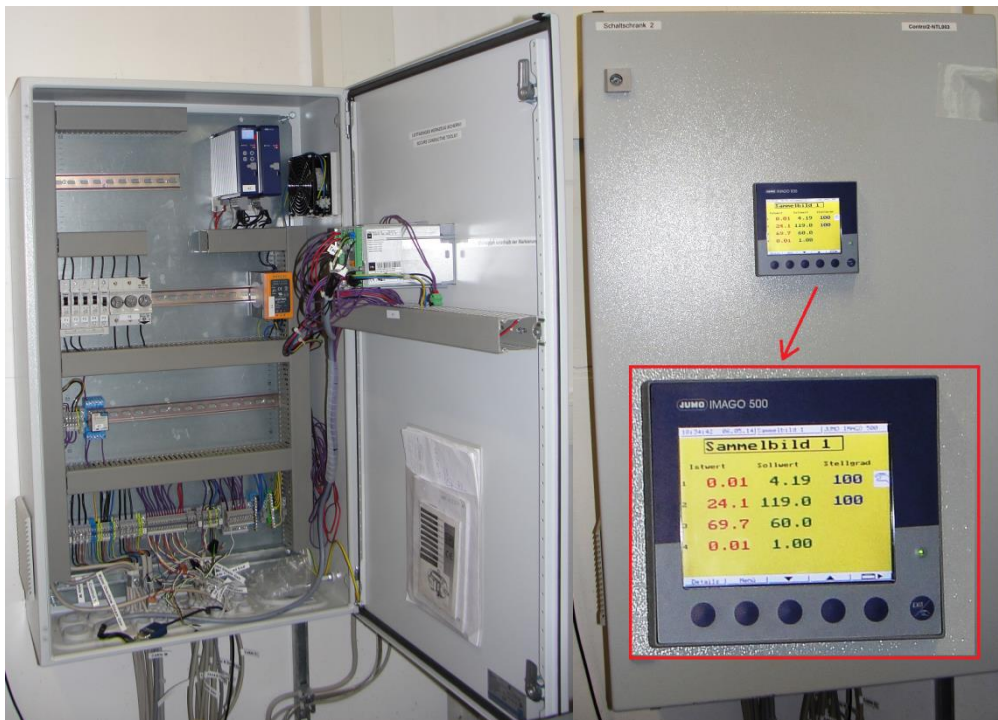
Figure 3.9 Electrical control unit 2. Left: Open, power thyristors can be seen at the upper-right corner. Right: The interface of the controller.
