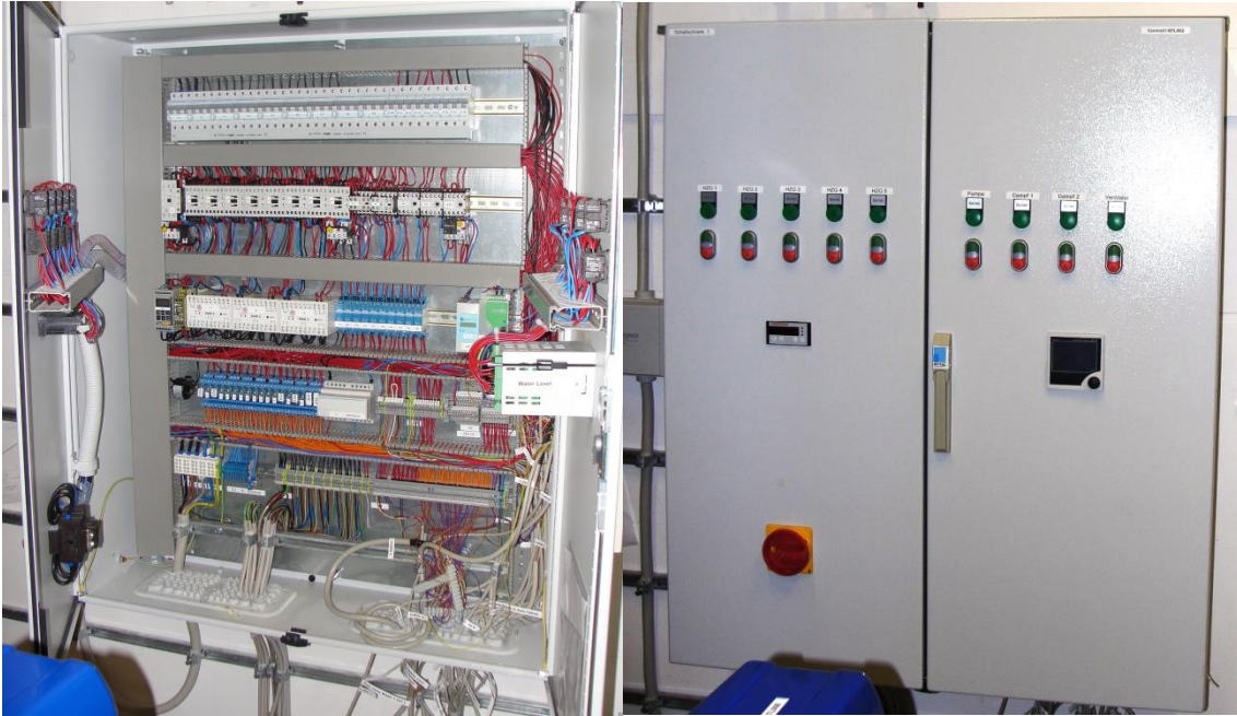
Figure 3.7 Electrical control unit 1. Left: open view with all components and internal connections. Right: closed view.
