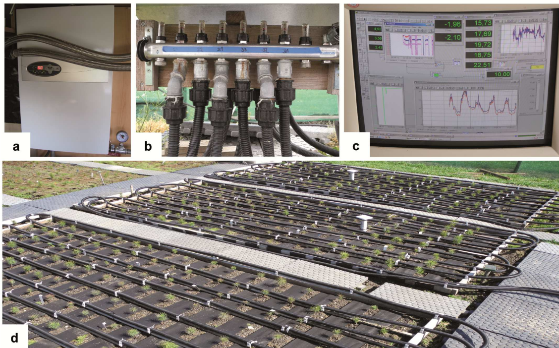
Figure 3.4 Heating system at the field experiment consisting of a) the boiler, b) the water distributor, c) the computer-control, d) the tubes and stripes of black, water-permeable geomembrane at the heated plots
