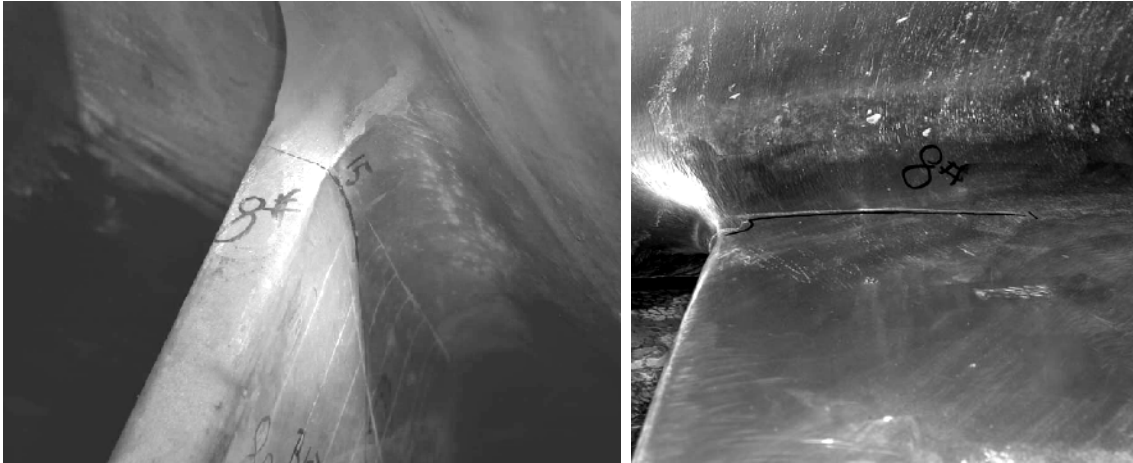
Figure 1.1: Typical fatigue cracks at the runner blade trailing edge, near to the crown (left) and near to the band (right).
