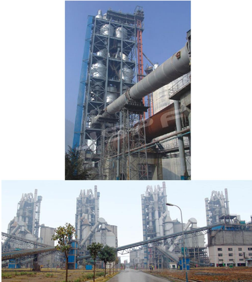
Figure 5: Modern cement rotary kiln production line with a daily output of 5,000 tons [obtained from Jiangsu Pengfei Group Co., Ltd]
