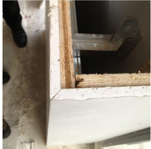
Figure 3: The insulation gap to be insufflated and covered by wood board and plaster board.
