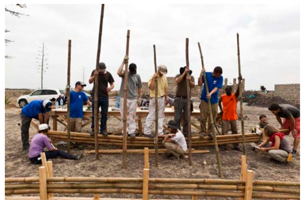
Figure 1: German and Kenyan students testing a prototype truss at the construction site in Kenya
