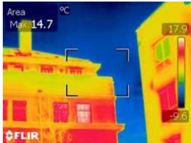
Figure 4: Infrared thermographic image of the Royal Standard House and Flat 30 on the upper floor.
